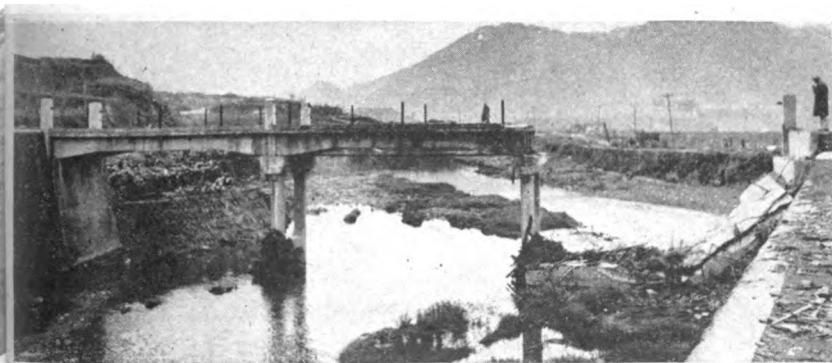
Figure 5.67c. Reinforced-concrete bridge with T-beam deck, 2,330 feet from ground zero. Part of deck was knocked off the pier and abutment by the blast, causing one span, 35 feet long, to drop into the river. The remainder of the bridge was almost undamaged.
